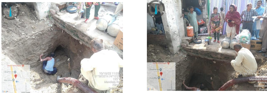
Figure 8: Leakage and Repairing at Water Supply lines MC Kamoke
