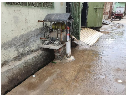
Private pumps have been common in the sub-project area due to under-demand or contaminated water supply.
