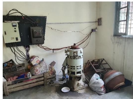
Condition of the Water Supply Infrastructure at Mandiala Water Works
