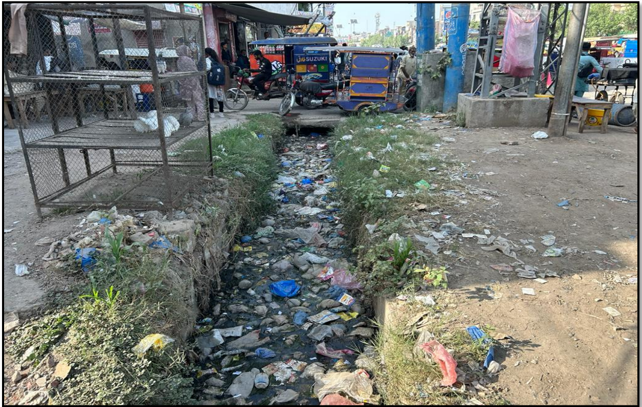
Fig. 1.5: A view of Drain clogged with solid waste
