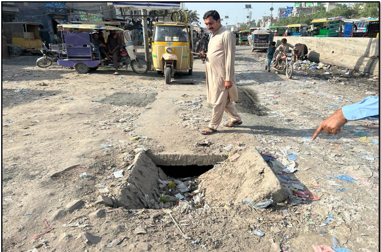
Fig. 1.6: A view of Drain, indicating damaged cover slab
